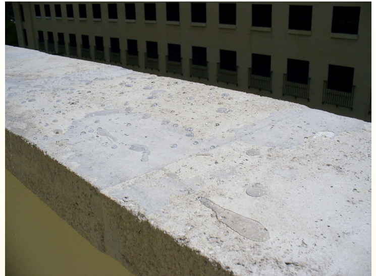
AFTER: Substrate chemically cleaned with CT-50 Remove and then sealed with a single coated PEN50 which penetrates deep into porous substrate. blocking the capillary action of water.
