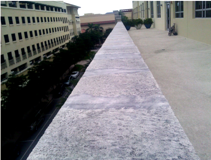
BEFORE : Porous stone substrate . Mold, Mildew Air-borne Dirt and Smog constantly leaving dirty appearance on building façade.
